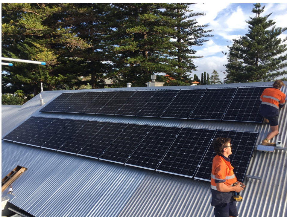
Figure 33. 6.4 kW PV array, Cottesloe
