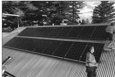
Solar panels are less conspicuous when they sit flat on a roof or are hidden behind a parapet wall
