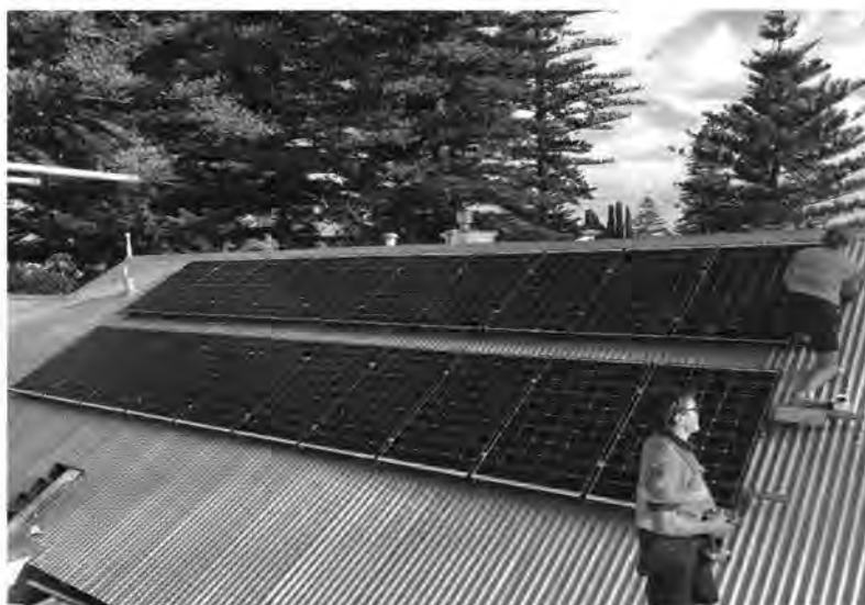
Figure 33. 6.4 kW PV array, Cottesloe
